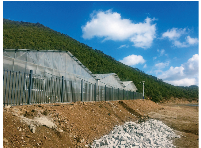
The Greenhouse of 1500 square meters for endangered medicinal plants built by Southwest Centre.
